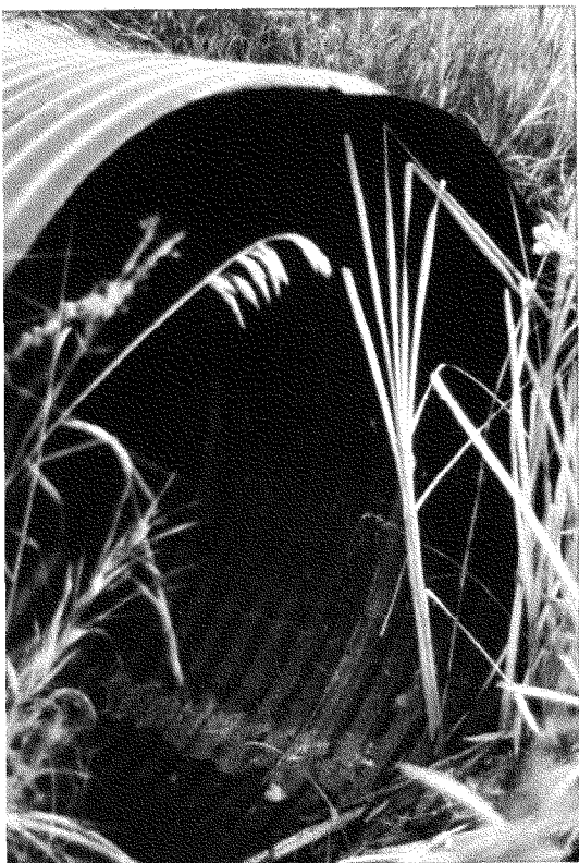
Installed more than 15 years ago in the western slope region of Colorado, this culvert under I-70 is in great condition.
