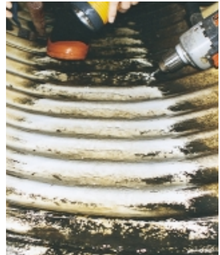
▲ This close-up view shows the Aluminized Steel Type 2 pipe installed in Garland, Maine, with the dark staining wiped away to reveal the like-new underlying aluminum.
