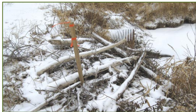
UPSTREAM END OF CULVERT THAT WAS CONSTANTLY PLUGGED BY NUISANCE BEAVERS
